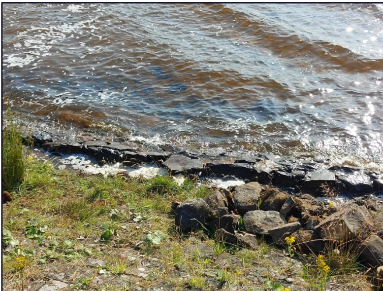
Fig2. The reservoir levels required to be dropped before repair works could commence.
