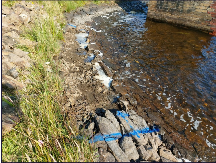
Fig 1. Existing pitch stones missing from the upstream reservoir wall.
